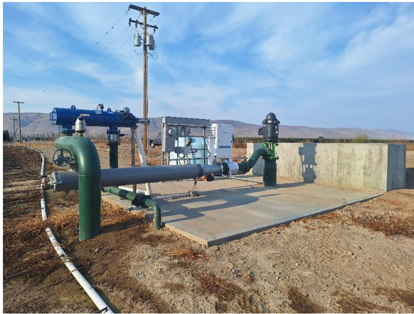
A pump station with a concrete water box and multiple filter systems for a pivot and drip system featuring a variable frequency drive.
